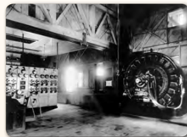
The first AC Generator
